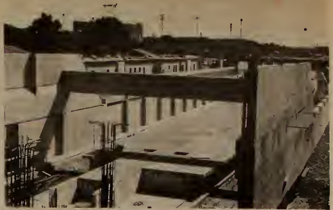
The site of the new Massachusetts Avenue station begins to take shape as part of Line Contract 097-115
